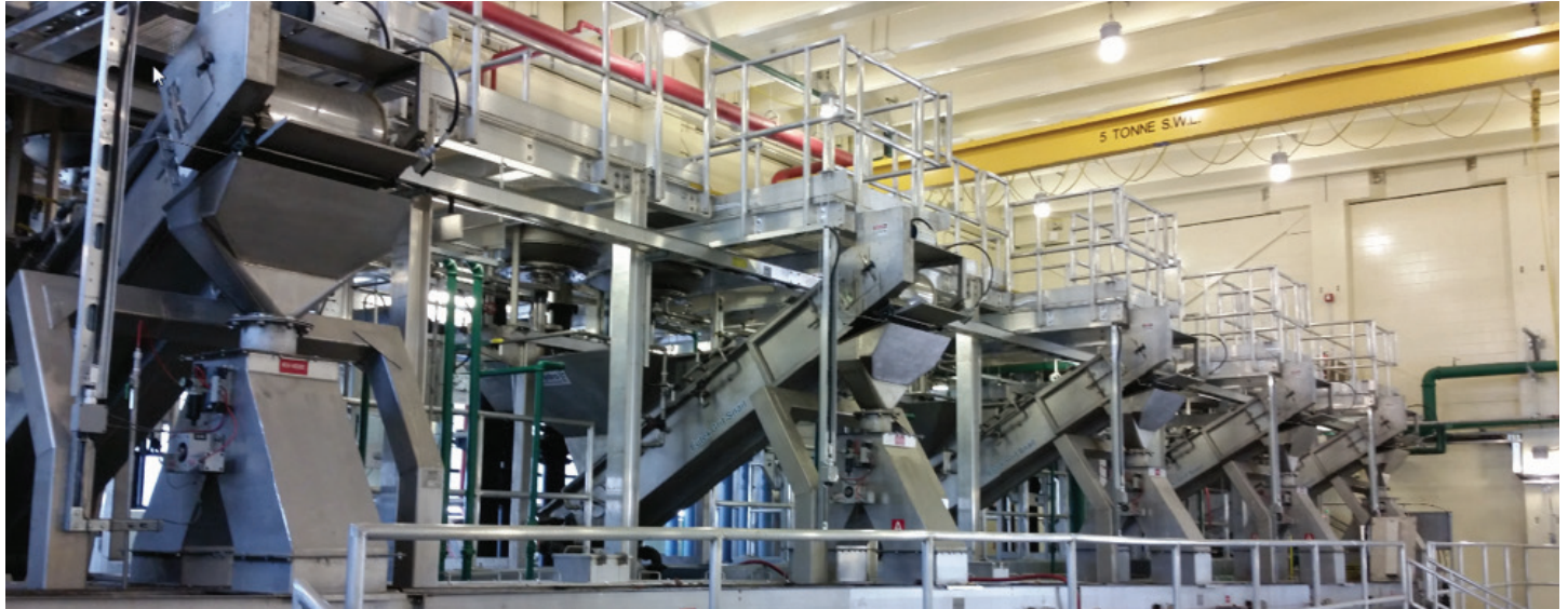
A high-performance grit removal system can significantly reduced downstream plant operating costs. Hydro International grit removal installation, Bonnybrook, Calgary, Canada
